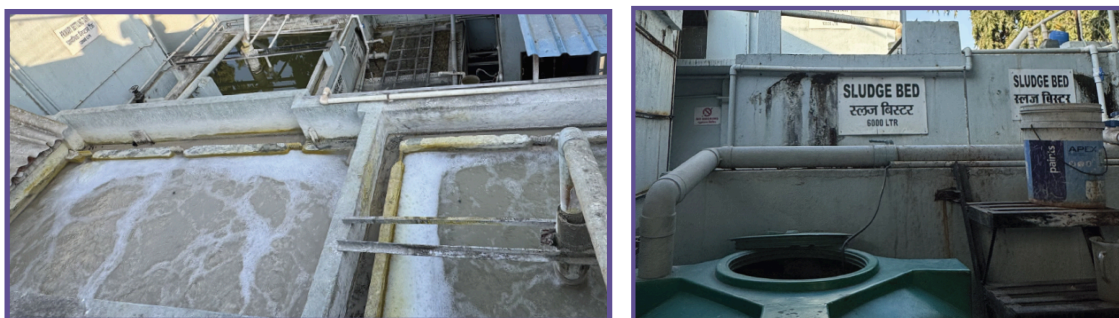
Figure 26: ETP at Neeman Carpets, Mirzapur
