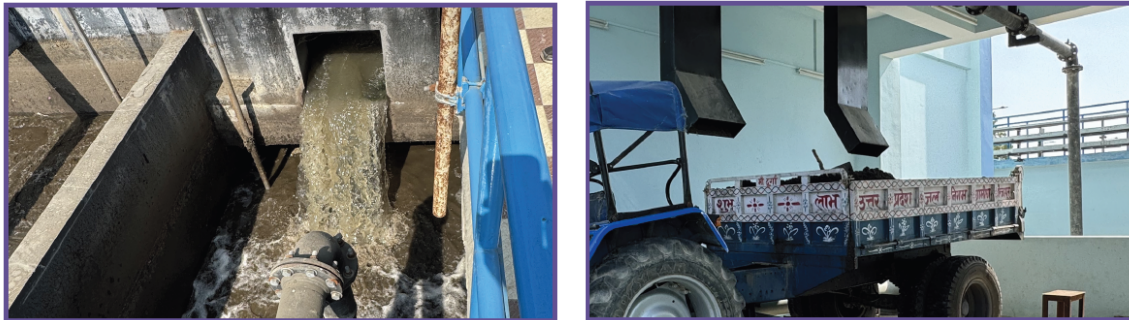
Figure 19: Inlet WW Chamber from Households and Transportation of Sludge
