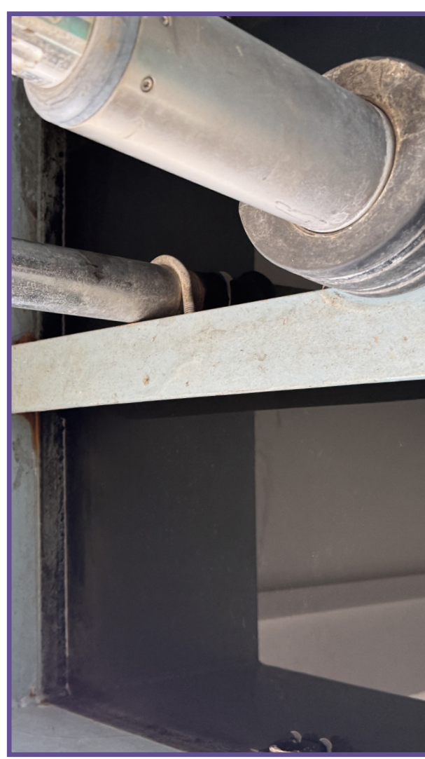
Outlet Water Chamber after Treatment
