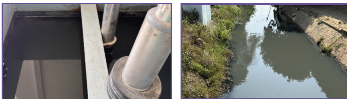
Figure 17: Outlet Water Chamber after Treatment and Open Outlet Drain from STP
