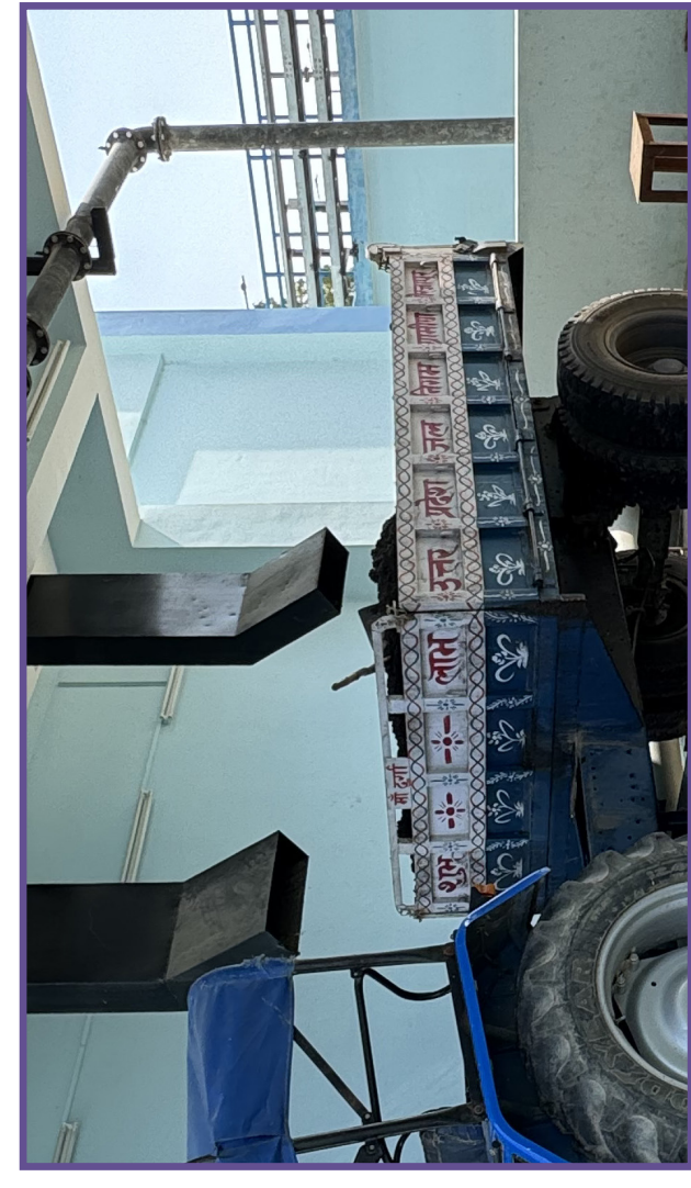
Transportation of Sludge
